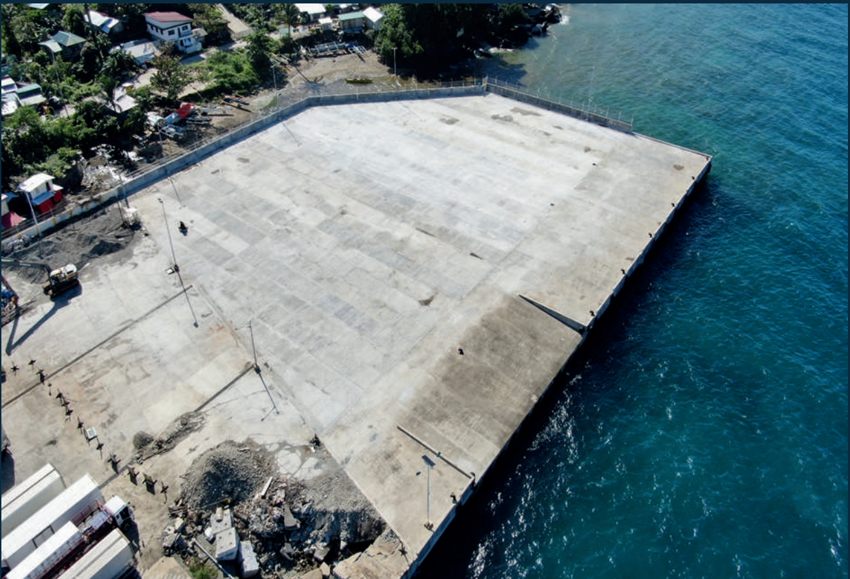
Expansion of Back-up Area with RORO Ramp at the Lipata Ferry Terminal
